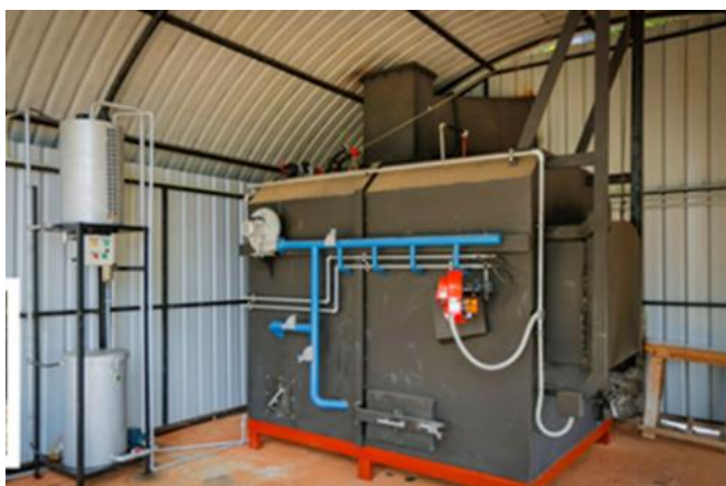
Incinerator installed in the DGH Chilaw
